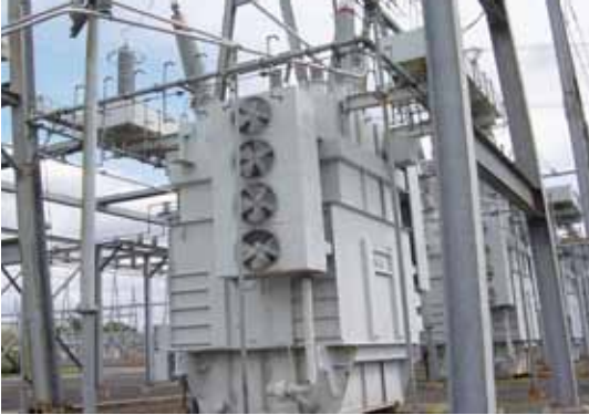
550 kV Transformer Line-Up
