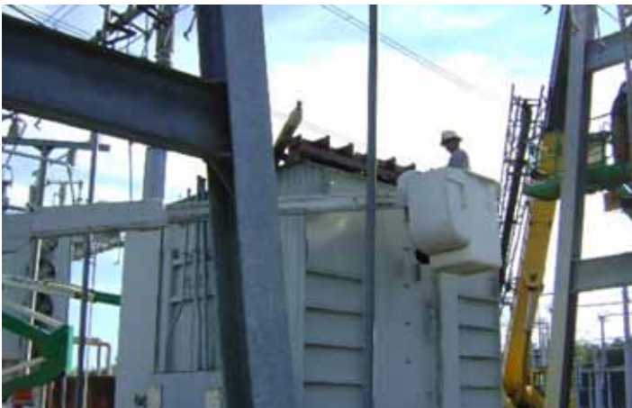
Transformer with Top Removed
